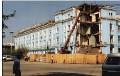
Fig. 12. Collapse of a corner of a building located in the centre of Yakutsk, 1999 (Photo by M. P. Grigoryev) (Alekseeva et al., 2007).
