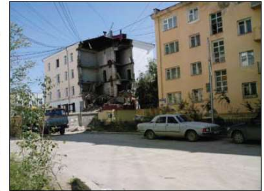
Fig. 13. Collapse of a part of the building belonging to the Administration for Geological Surveys in Yakutsk, 2009 (Photo by M. P. Grigoryev)
