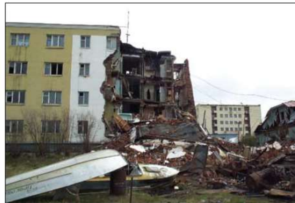
Fig. 14. A building section collapsed due to weakened basement, Chersky village. (Photo by V. E. Romanovsky)
